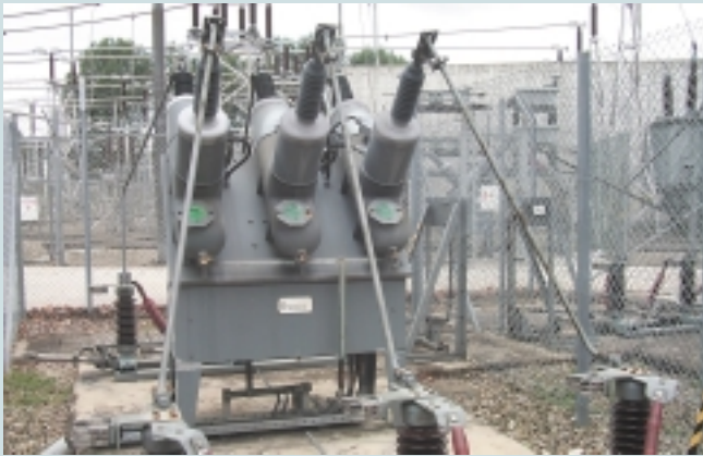
33kV Circuit Breaker with 200kV dc High Voltage Power Supply in the background
